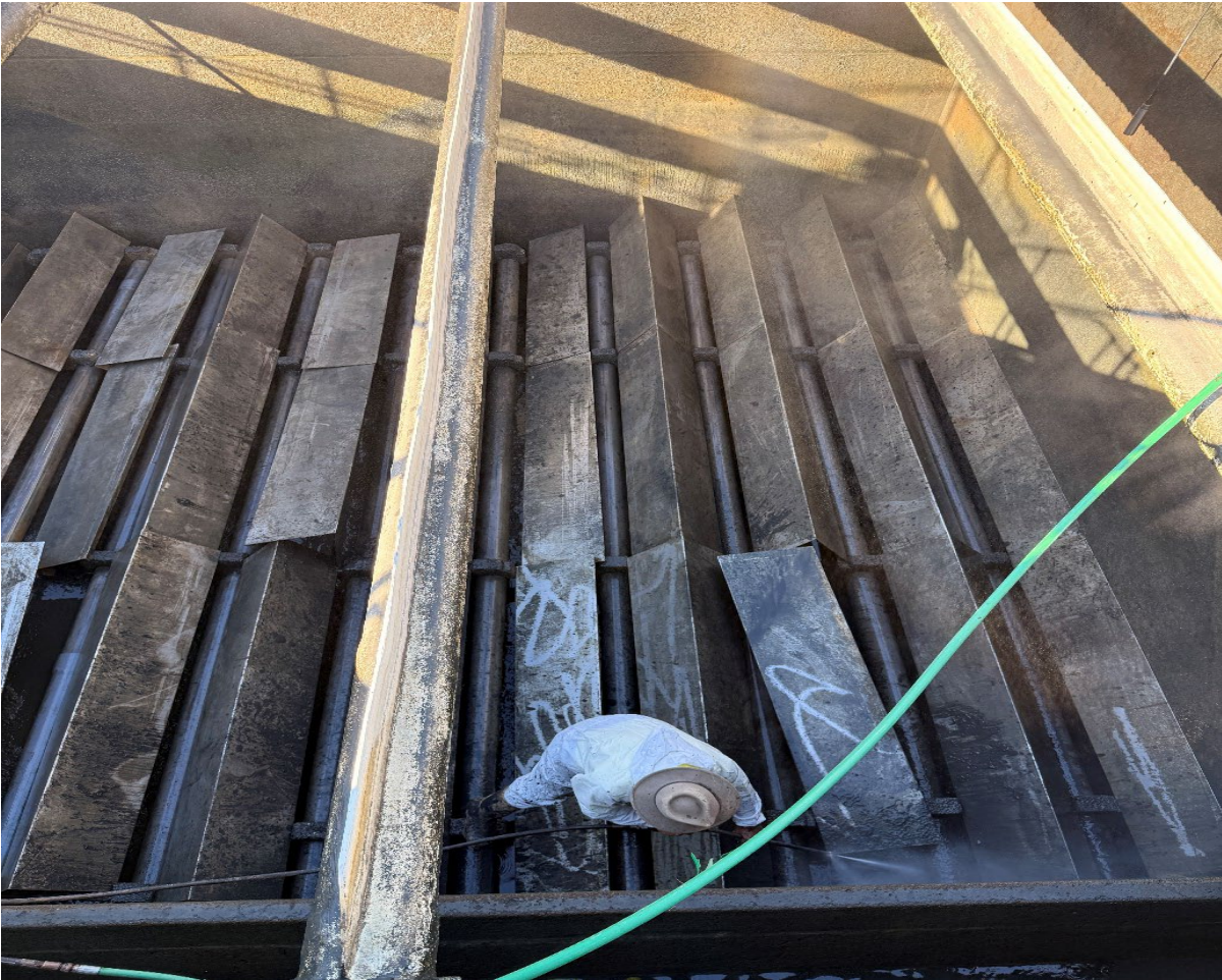
clarifier wash out at water treatment plant
