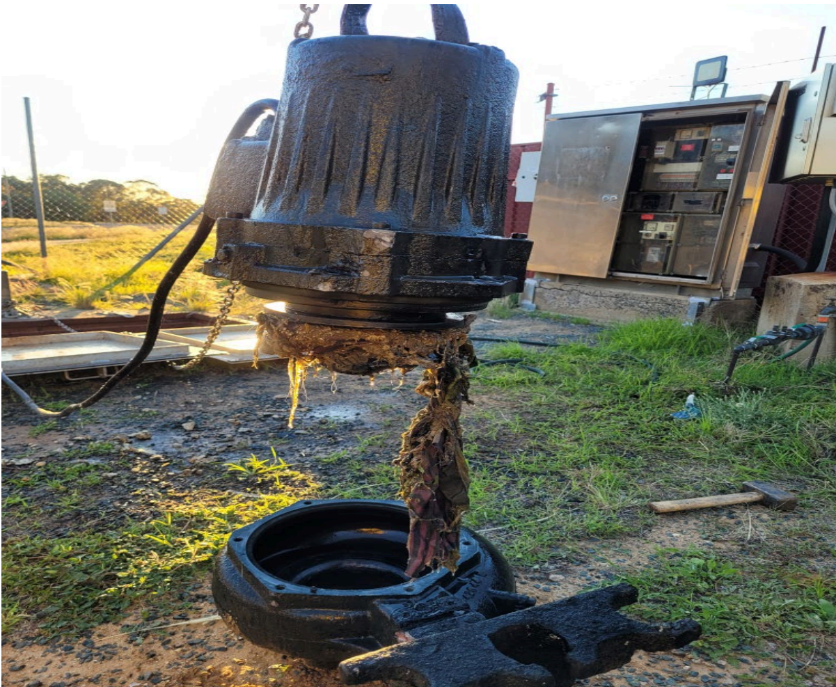
Lang street sewer pumping station – ragging
