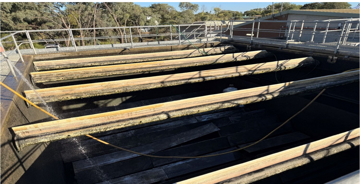
clarifier wash out at water treatment plant
